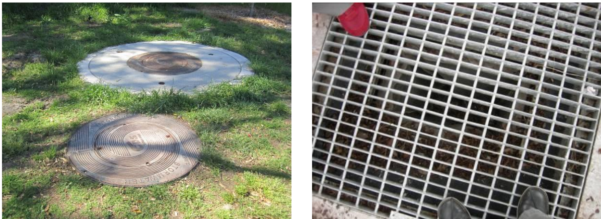
Figure 4: GPT in Centennial Park (left), inlet basket (right) (Photos: Alluvium)
