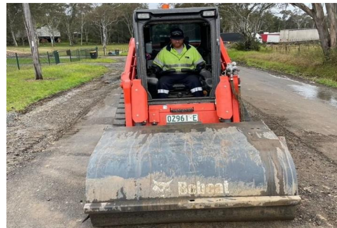
Council staff member assisting in flood recovery efforts.
