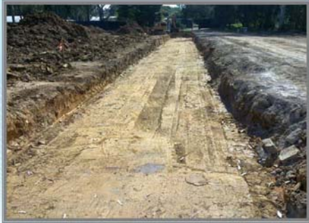
Foundation works for the dam wall for the Jardine Drive flood detention basin.
