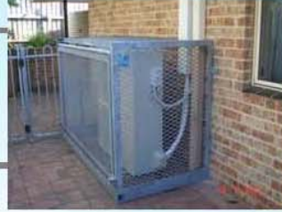
Air conditioning unit installed at Holsworthy Childcare Centre
