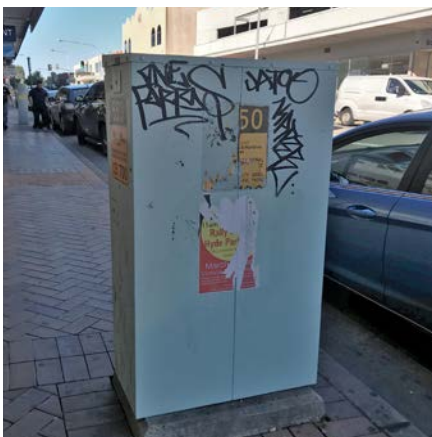
Figure 8.420 Detail of street electrical box on the southern side of Scott Street.
