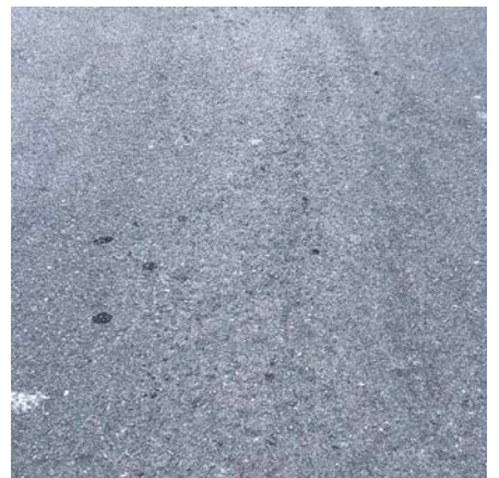
Figure 8.432 Detail of pavement on Norfolk Serviceway's. Near the intersection with Bathurst Street.
