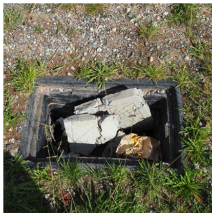
Figure 8.334 Collapsed electrical cap detail. Bigge Street, east side.
