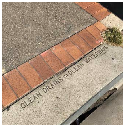
Figure 8.429 Detail of Road Drain, located at Norfolk Serviceway northern entrance, next to Memorial Avenue.
