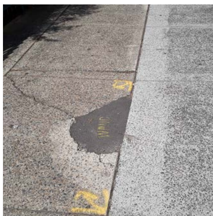
Figure 8.358 Detail of pavement of George Street's western side. In the middle of the street between Campbell Street and Elizabeth Street.
