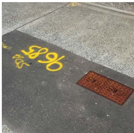
Figure 8.354 Detail of pavement of George Street's eastern side. Close to Campbell Street.
