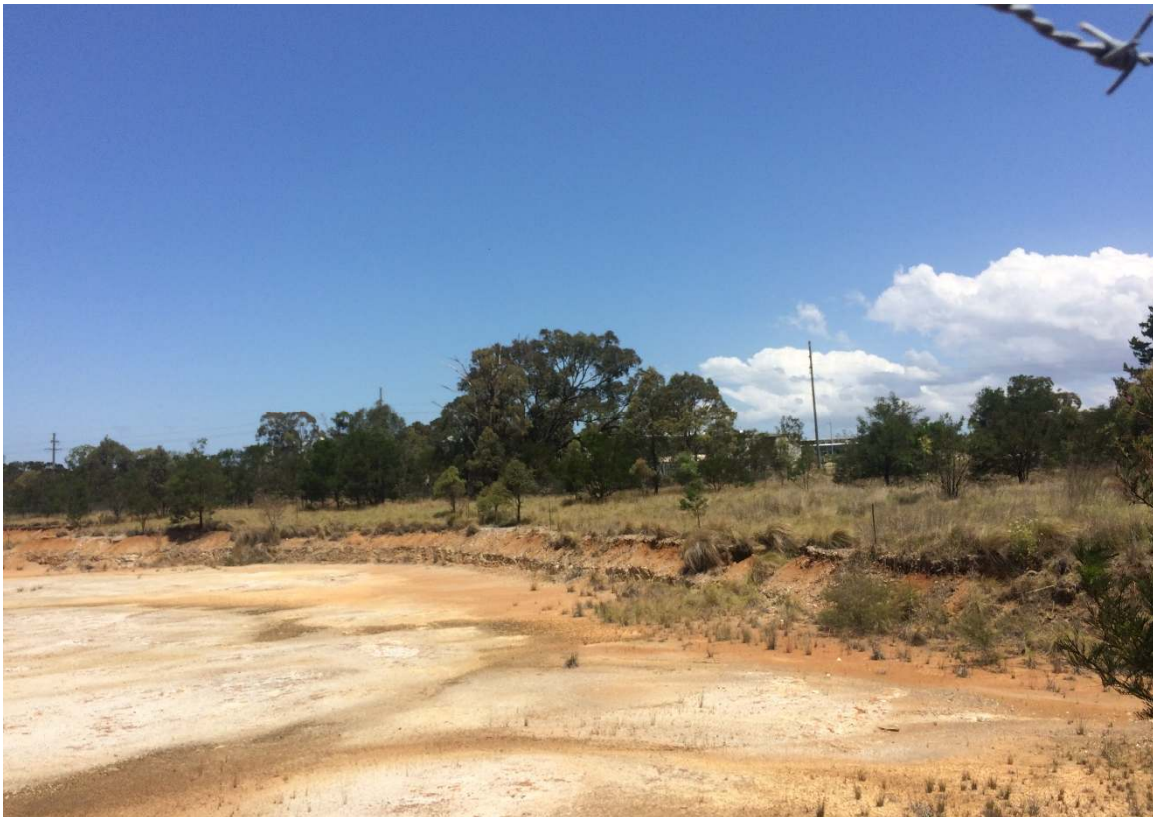
Photograph 2 – Excavated and compacted gravel on the midsection of the site (Southern view).
