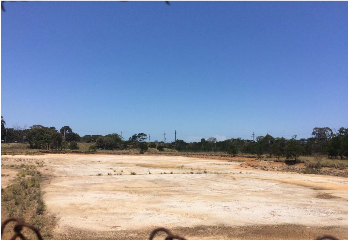
Photograph 1 – Excavated and compacted gravel on the midsection of the site (Eastern view).
