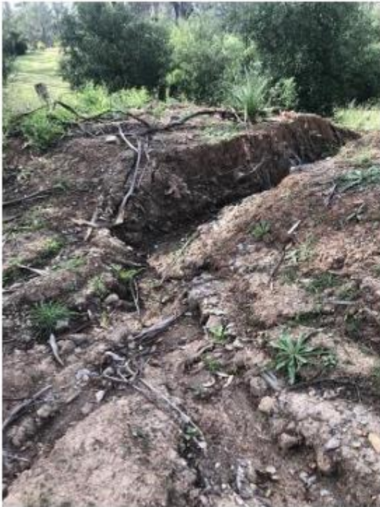
Image 9 - Compromised bunding wall in North-Eastern corner resulting in sediment laden water being discharged onto adjoining property
