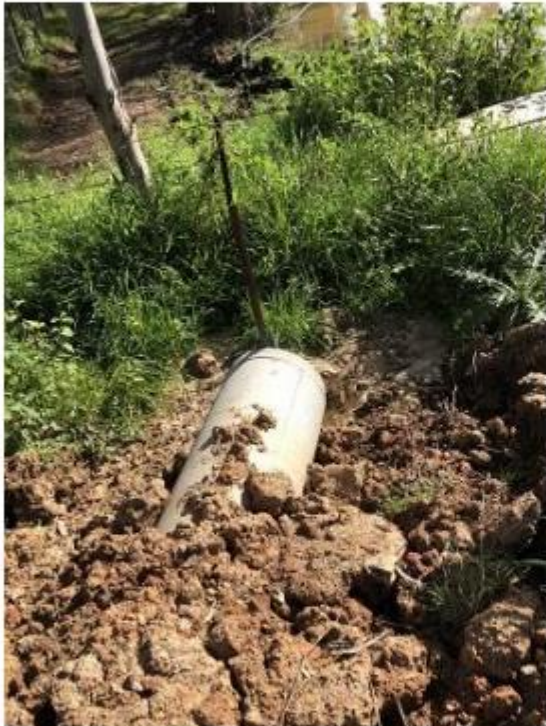
Image 10 - Outlet pipe positioned to discharge into neighbouring premises adjacent to their dam
