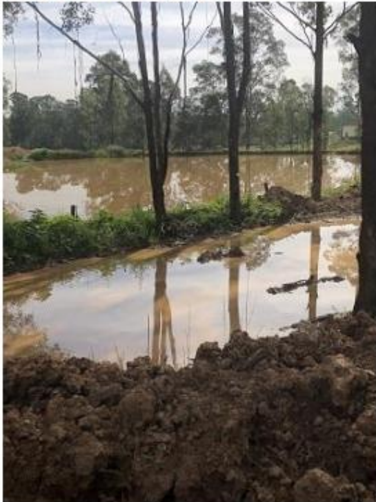
Image 8 - Absence of/ or inadequate sediment control measures resulting in sediment laden water being discharged into dams on adjoining properties
